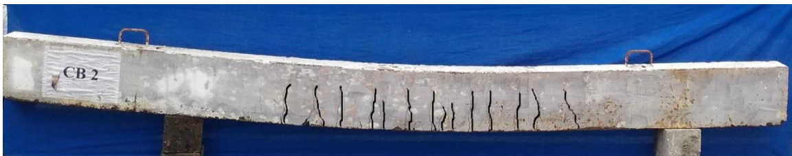
Fig. 12 Crack Pattern of CB2
