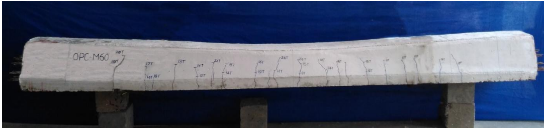
Fig.10 Crack pattern of OPC Sleeper
