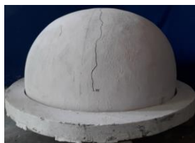
Fig. 11 Crack Pattern of Dome
