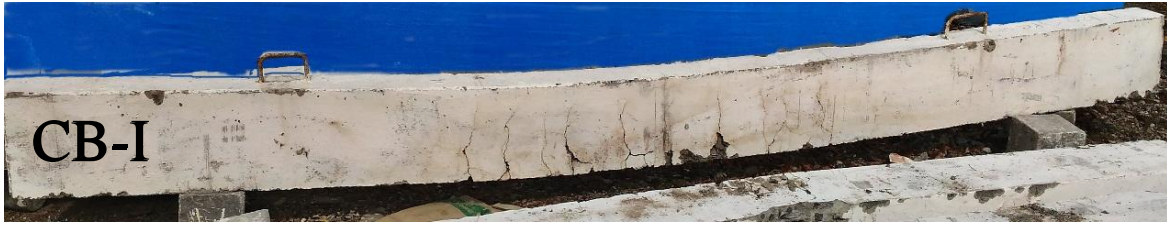
Figure 24 Cracking Pattern of Control Beam Under Static loading
