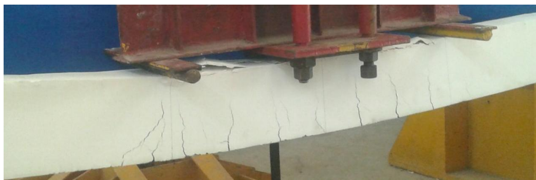
Fig.14 Crack Pattern of GB2
